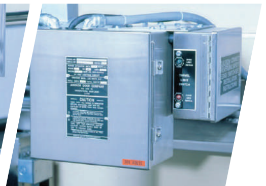
NEMA 4X Control Panel
